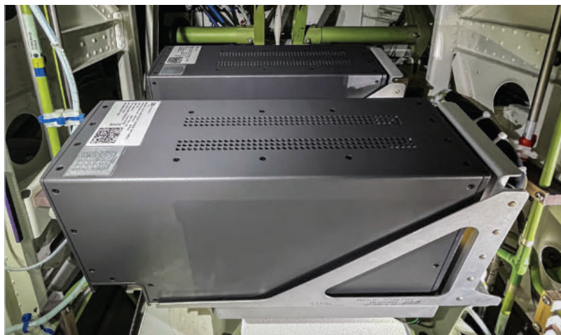
SD Plane Simple® Ka-Band & Ku-Band modems (SMUs) installed in the non-pressurized area of a G550
