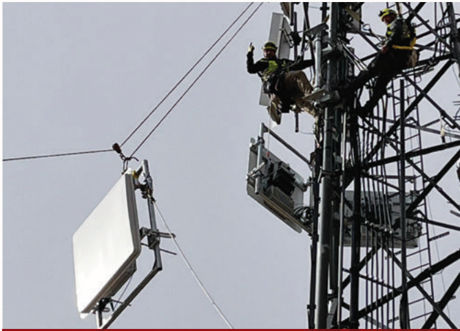
Colorado - 5G antenna install
